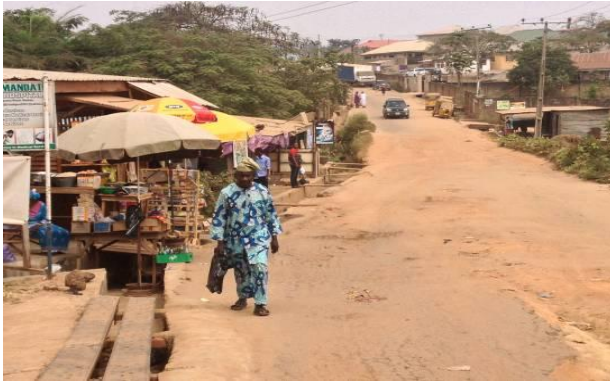
e.) Affected kiosks along the drainage way damaged bridge
