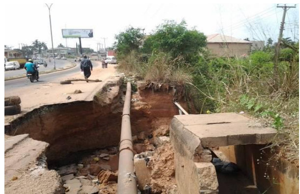
d.) Collapsed outlet fast eroding
