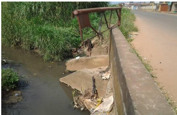
Structural damage to existing culvert
