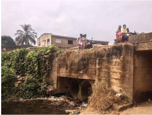
Collapsed culvert with debris
