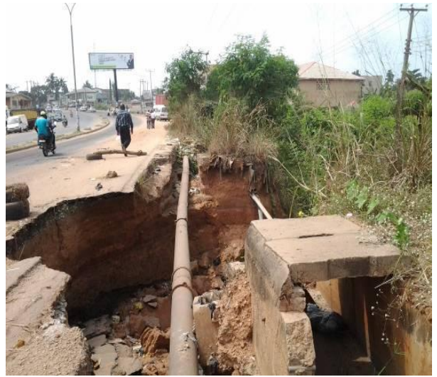
d.) Collapsed outlet fast eroding
