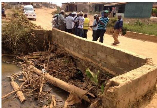
Pipe culvert blocked by debris
