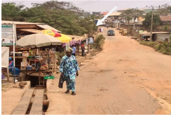
e.) Affected kiosks along the drainage way damaged bridge
