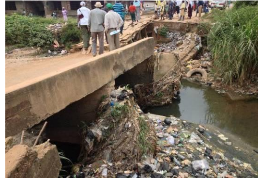
Debris collects against a collapsed structure
