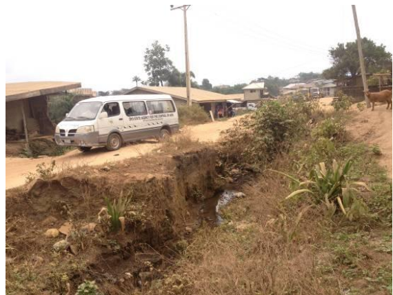
Collapsed culvert and road approaches without
