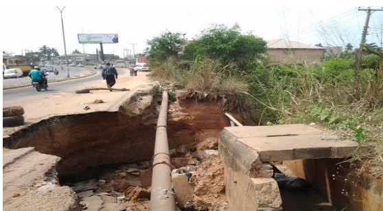
Undercutting of road; damaged drainage
