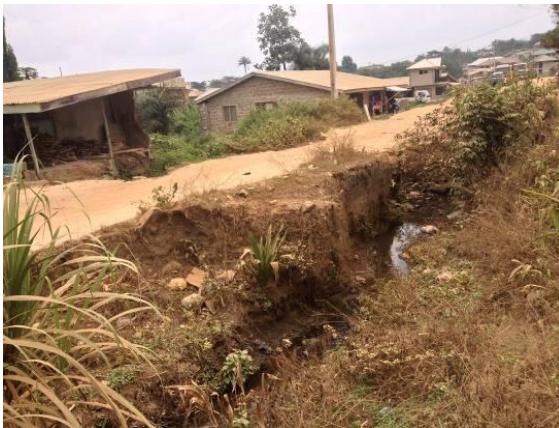
Collapsed culvert drainages
