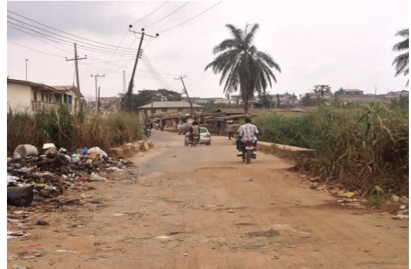
Damaged road approach;
