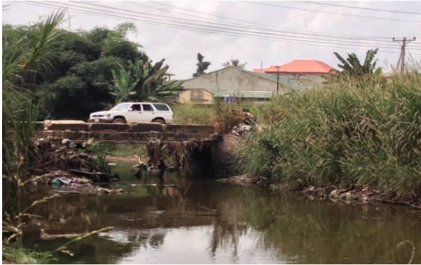
View from downstream; aquatic weed/manmade improper solid wastedebris restricting flow of water
