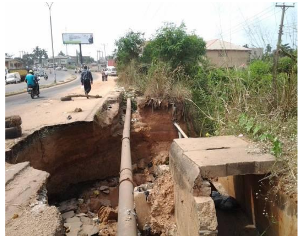
d.) Collapsed outlet fast eroding
