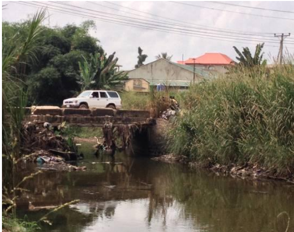
View from downstream; aquatic weed/manmade debris restricting flow of water
