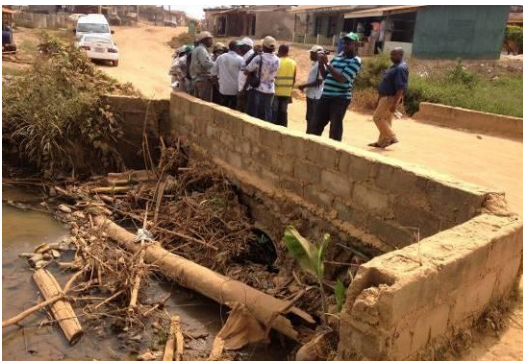
Pipe culvert blocked by debris
