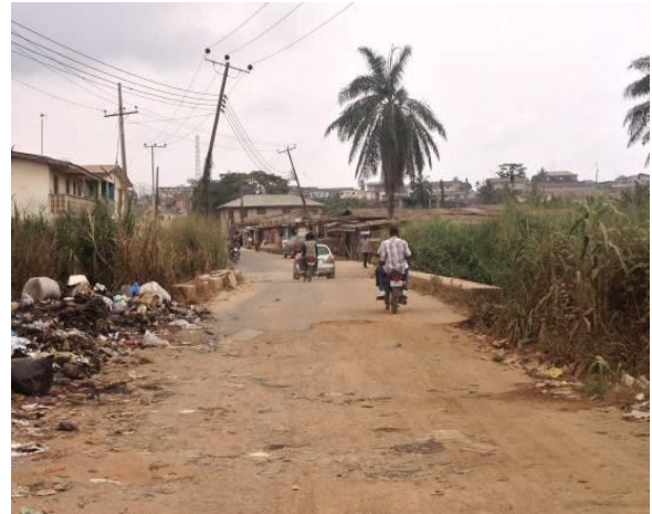
Damaged road approach; improper solid waste
