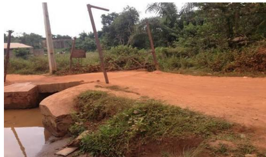
Inadequate single culvert
