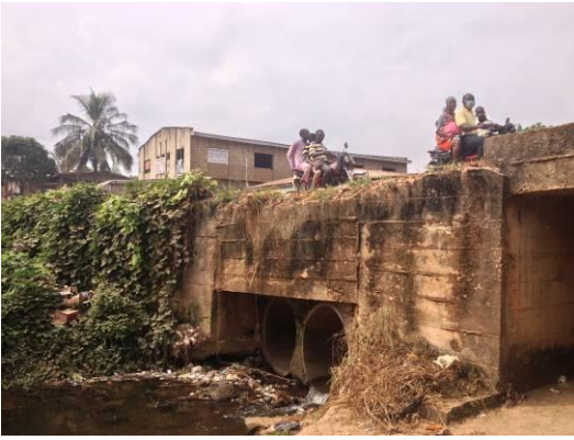
Collapsed culvert with debris
