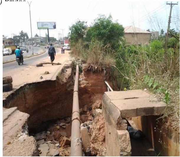
d.) Collapsed outlet fast eroding
