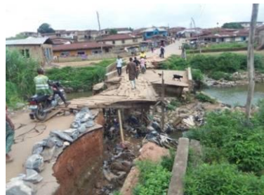
A section of damaged culvert showing existing damaged
