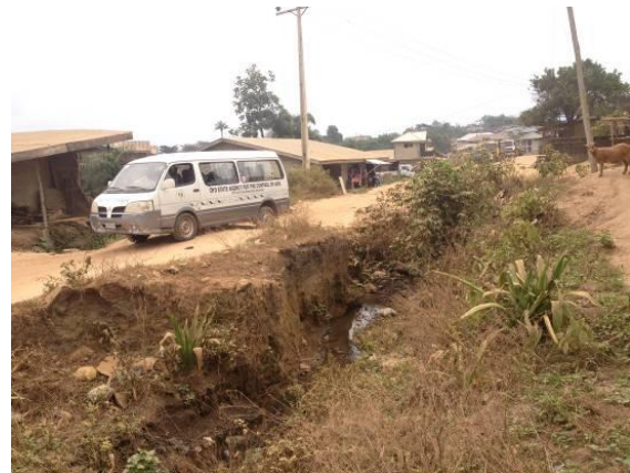
Collapsed culvert and road approaches without drainages
