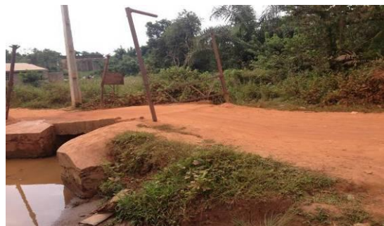
Inadequate single culvert
