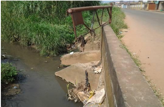
Structural damage to existing culvert
