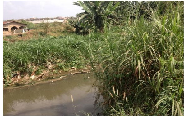
Aquatic weeds restricting flow of water
