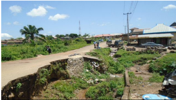
Eroded road drains with reinforce embankment by the communal efforts
