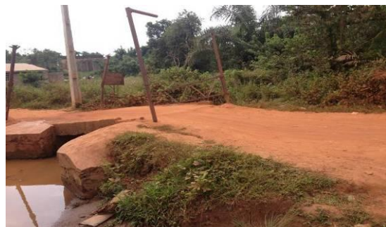
Inadequate single culvert
