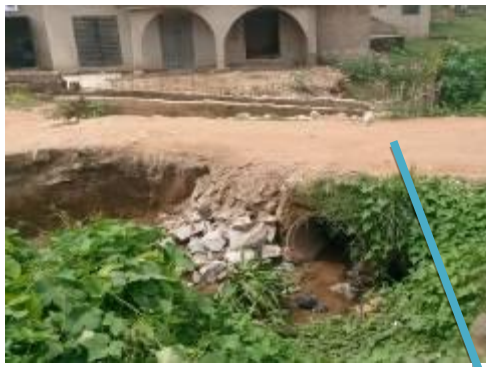
Inadequate existing ring culvert
