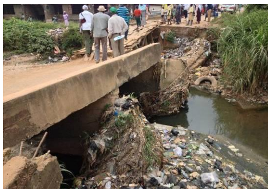
Debris collects against a collapsed structure
