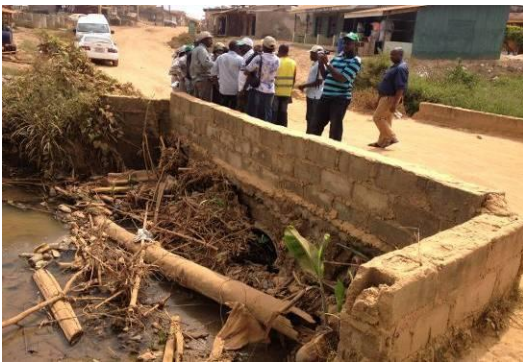
Pipe culvert blocked by debris
