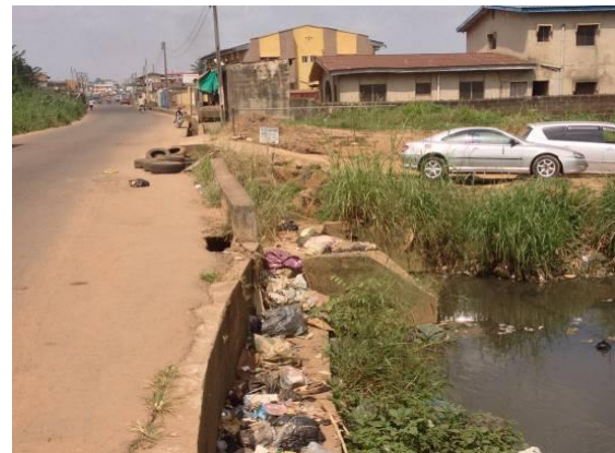
Turbid surface water; existing drainage as dump site
