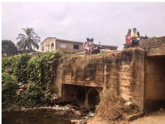
Collapsed culvert with debris
