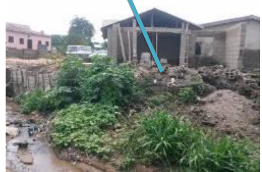
Dilapidated structure very close to stream
