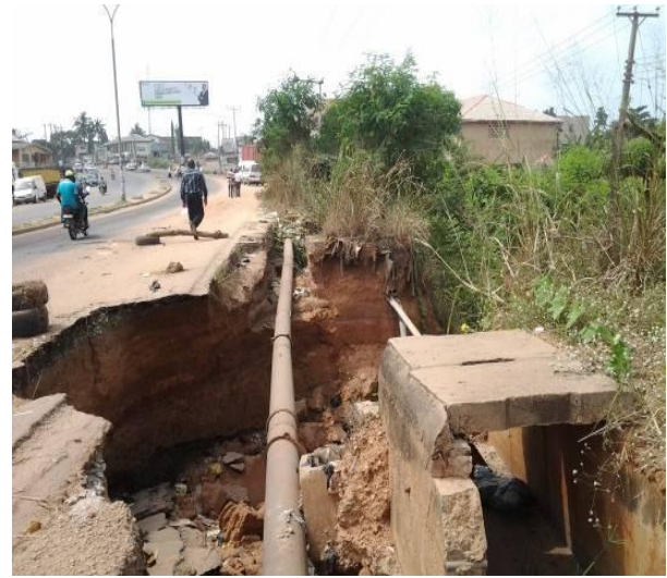
d.) Collapsed outlet fast eroding
