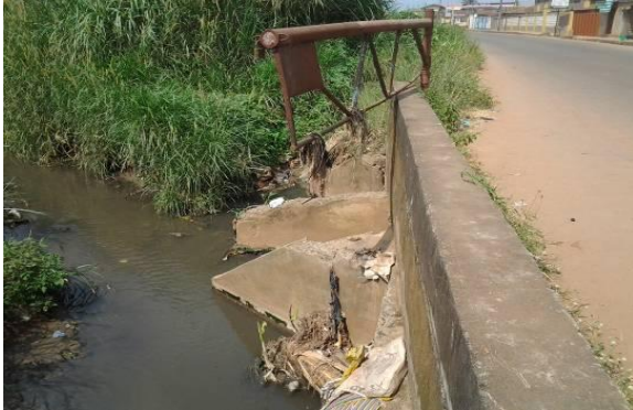
Structural damage to existing culvert
