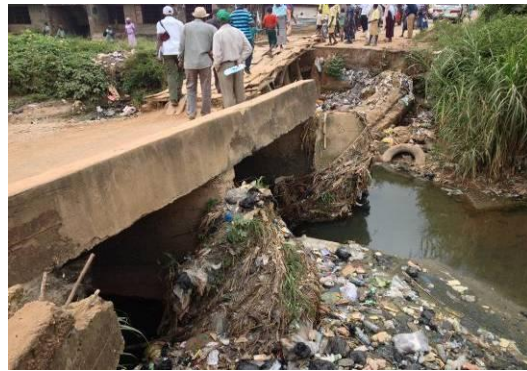
Debris collects against a collapsed structure
