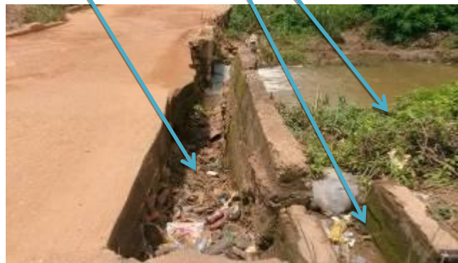
Part of the road being affected by flood, existing damaged drainage system and downstream vegetation
