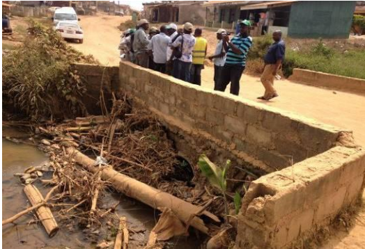
Pipe culvert blocked by debris
