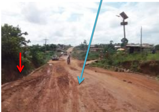
Egbeda Tuba road after damaged culvert leading to Elere community (foreground); and existing drainage systems
