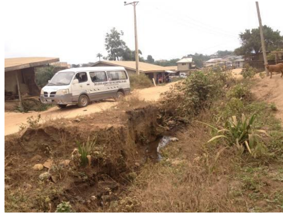
Collapsed culvert and road approaches without drainages
