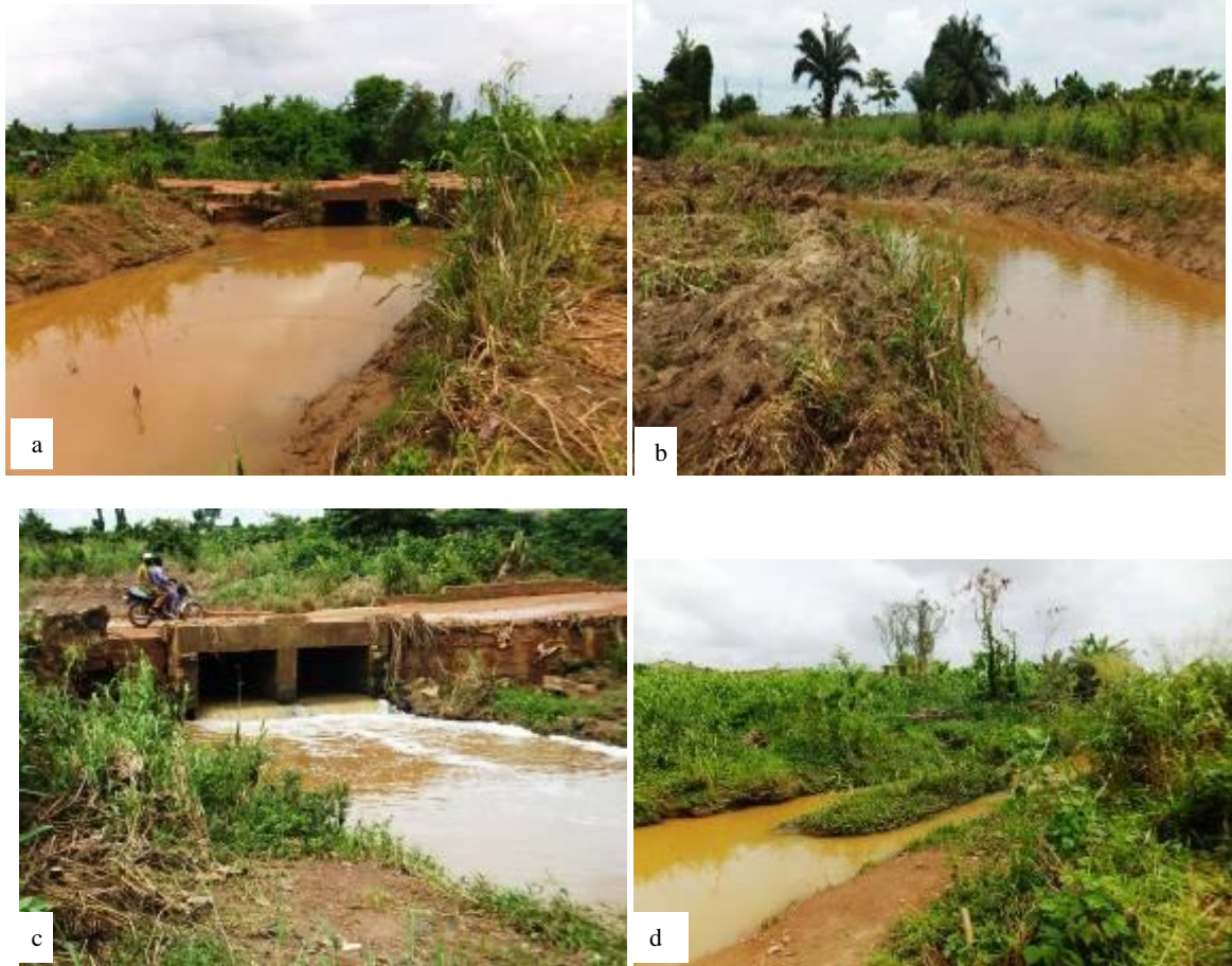
Plate 5.1(a-d): vegetation around Foworogi culvert
