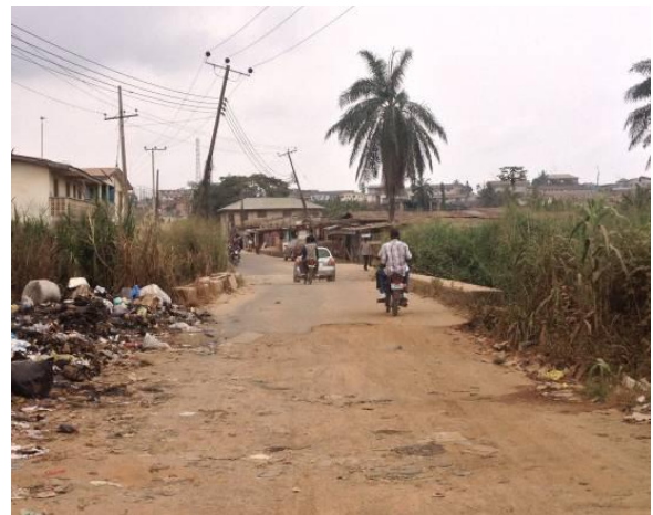
Damaged road approach; improper solid waste
