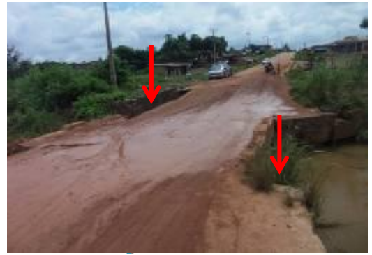
Damaged Foworogi culvert and part of the road being affected by flood
