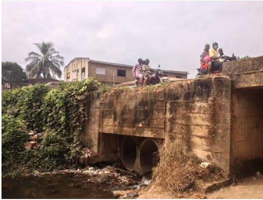
Collapsed culvert with debris
