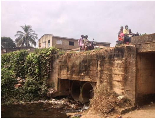
Collapsed culvert with debris
