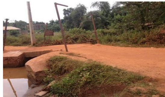
Inadequate single culvert
