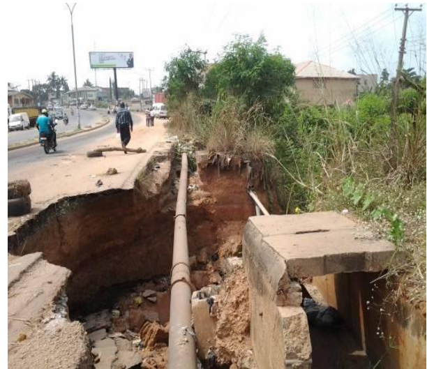
d.) Collapsed outlet fast eroding
