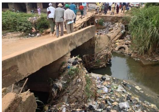
Debris collects against a collapsed structure
