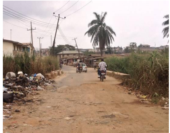
Damaged road approach; improper solid waste
