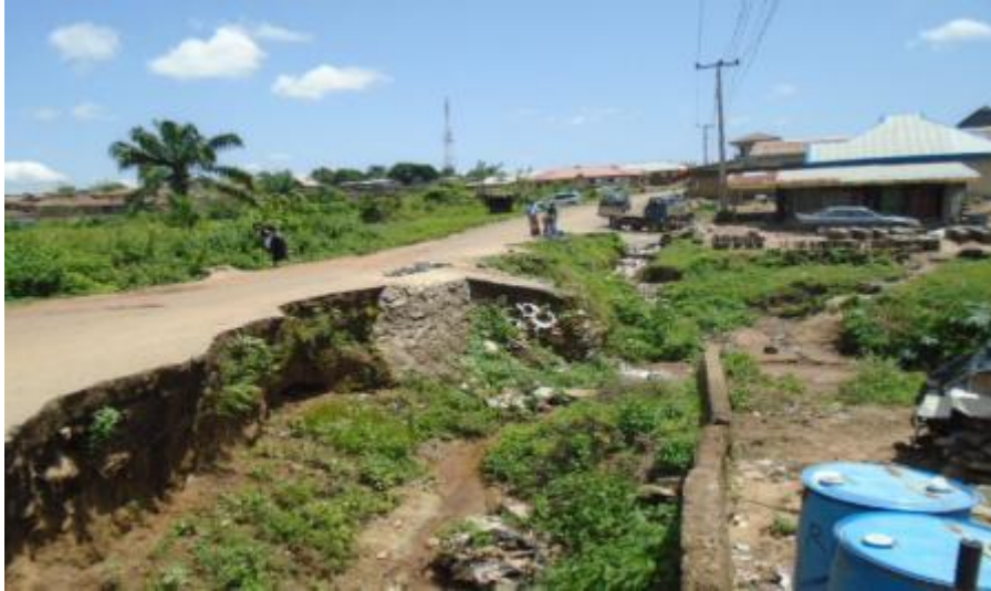
PIC 2.2: Massively Eroded Drainage
