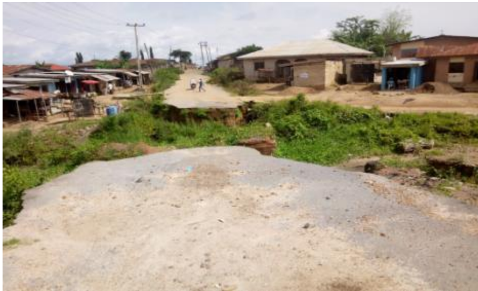
PIC 3.1 – Completely Damaged Culvert
